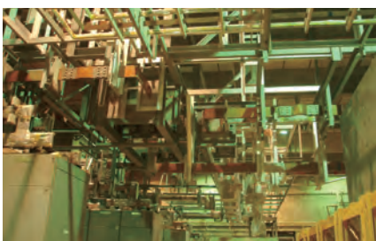
Transmission lines in the laboratory
