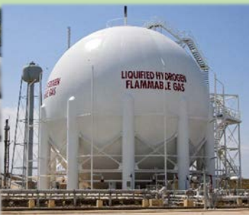
Liquid hydrogen storage (heavy)
